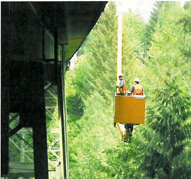
Steve Lovejoy, Senior Mechanical Engineer (left), and Nathan Leung, student intern, were suspended about 150 ft above the ground in a three-ft by three-ft bucket from which they placed postage-stamp size strain gauges.
